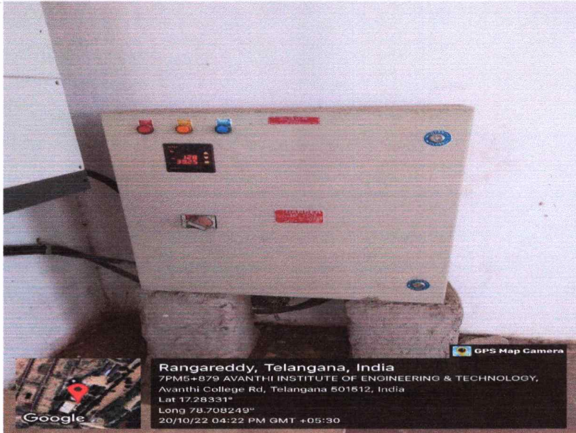
BLOCK-II Solar plant connected to power grid
