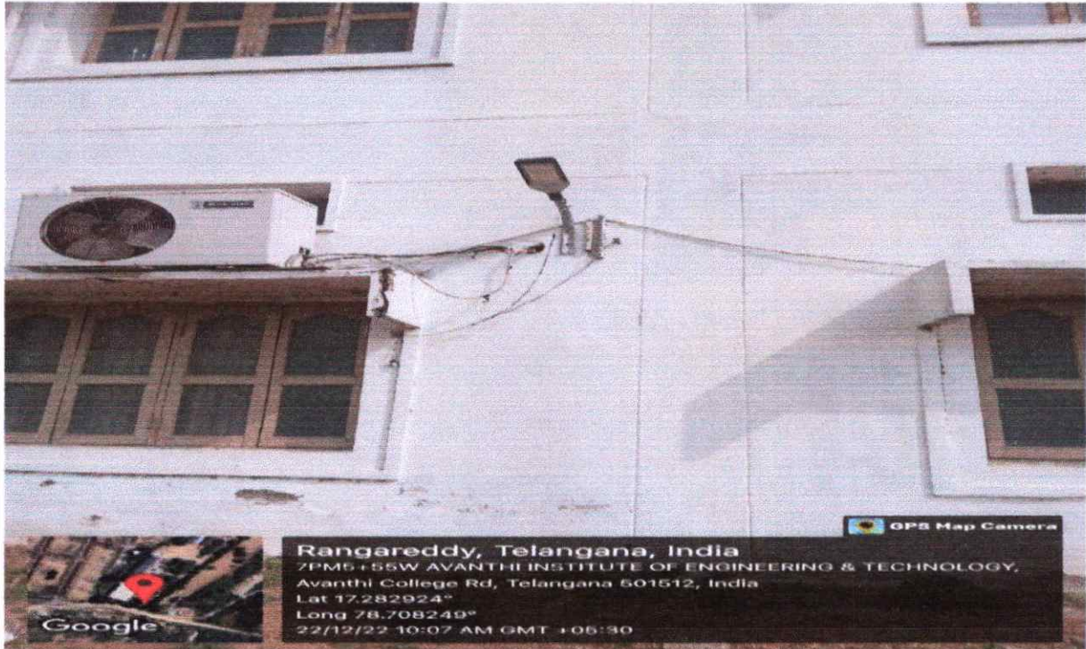
Installed LED lamp in the outside premises like corridors
