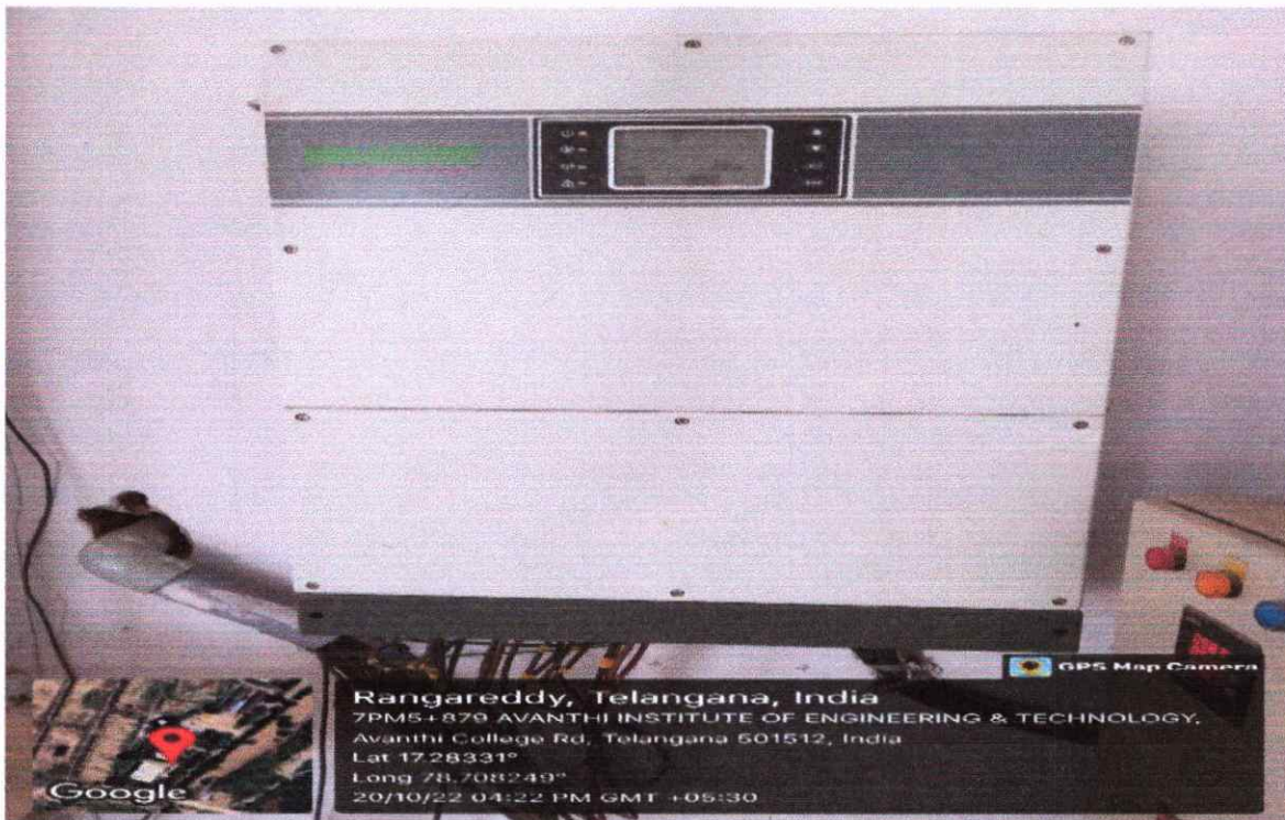
BLOCK-I Solar plant connected to power grid
